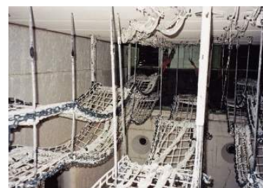
After the test Defem system after 90 minutes of fire test. The electrical performance is still intact.
